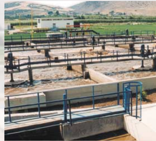
Third degree treatment of wastewater for the city of Levadia
