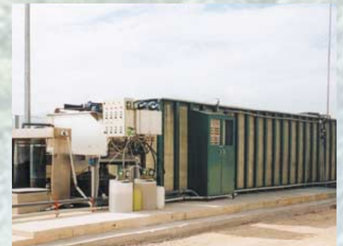
Autonomous Paper Mill Treatment Unit
