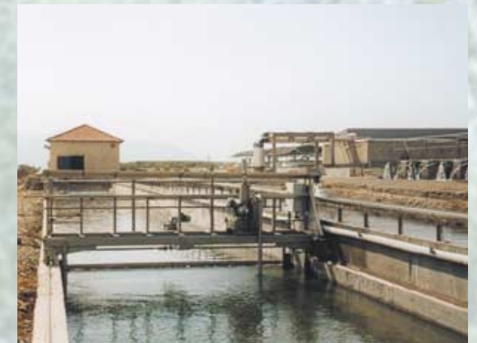
Fish Farm Effluent Treatment Plant
